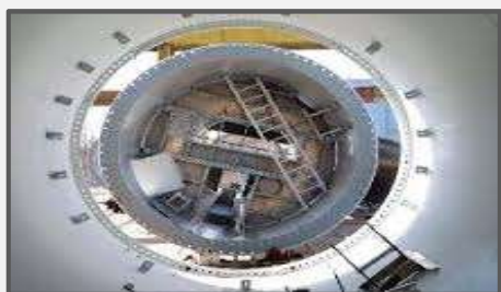
Tower Internal Parts
