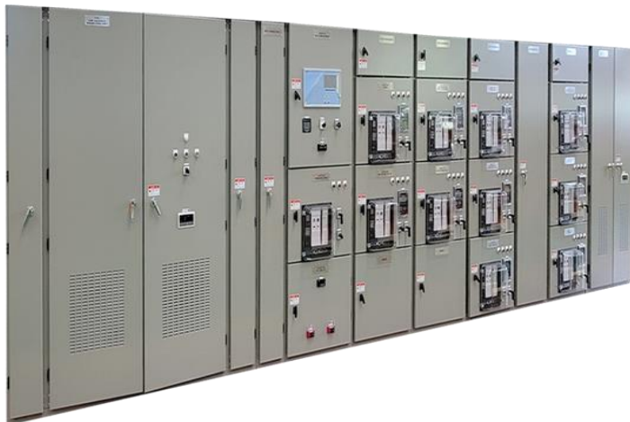
480V,5000A Low Voltage MCSG
